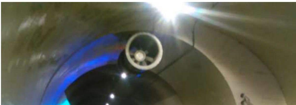
Sl.10 – Ventilator u tunelu
